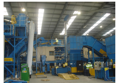
Materials Recovery Facility (MRF) at Longley Lane in South Manchester
