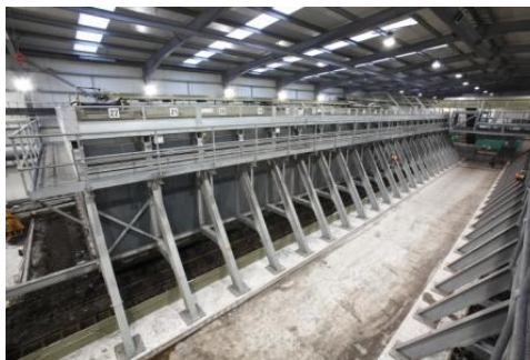
In-Vessel Composting Facility (IVC), there are currently three with a fourth coming on board next year.
