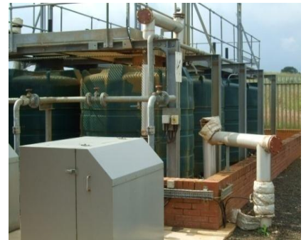
Methane Stripping Plant, at Adswold former landfill in Stockport
